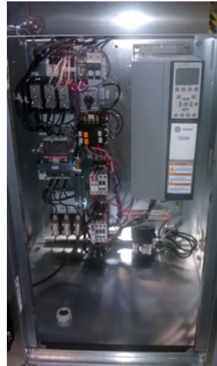
Figure 86. Internally mounted VFD
