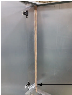
1 5/8-in. ± 1/8-in. gap between pipe cabinet and horizontal deflector
