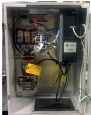
Figure 143. Externally mounted VFD
