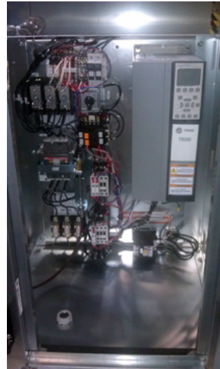
Figure 140. Internally mounted VFD
