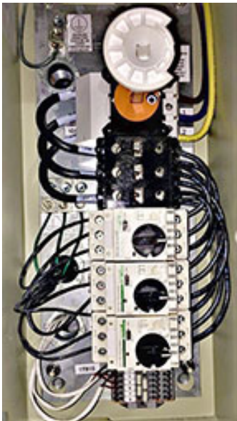
Figure 142. External motorized impeller control panel (MICP)
