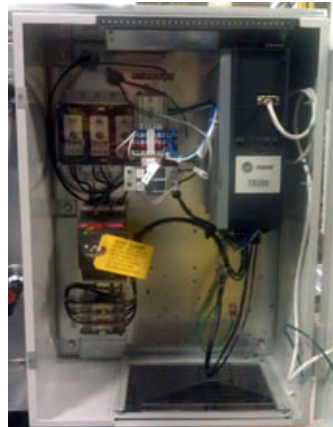
Figure 15. Externally mounted VFD
