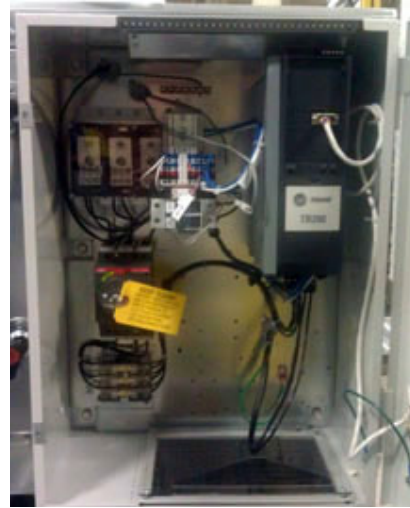
Figure 83. Externally mounted VFD
