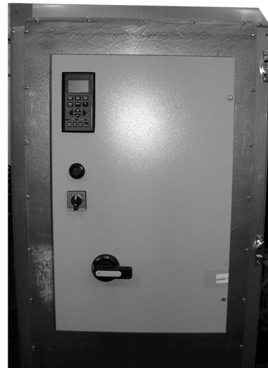
Figure 60. Variable-frequency drive (VFD)
