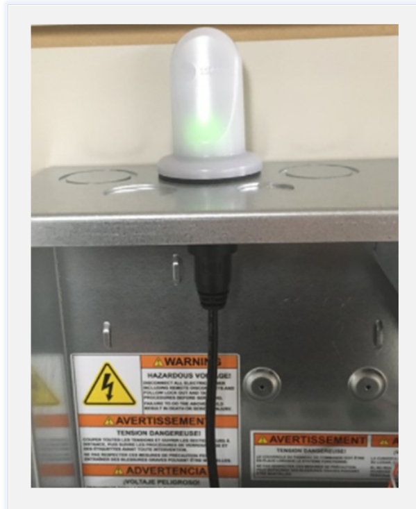
Figure 48. Trane USB Wi-Fi Module installed in the Tracer SC+ panel
