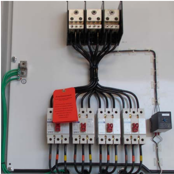
Figure 23. Power distribution panel
