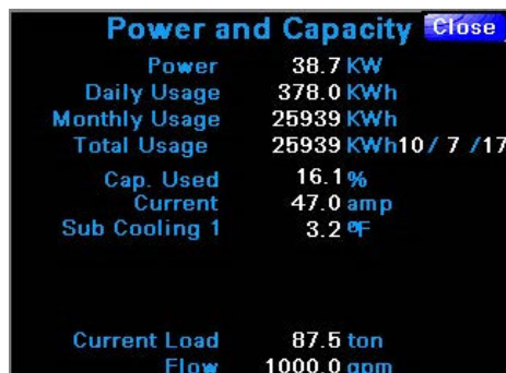
Figure 19. Power and capacity control screen
