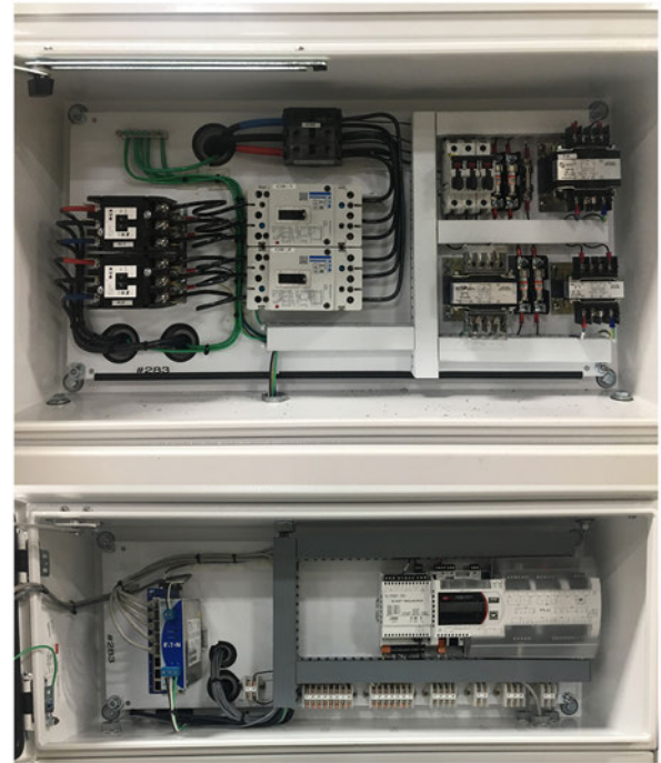
Figure 27. Module electrical panel
