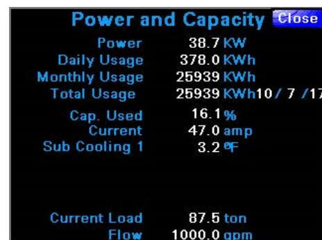
Figure 25. Power and Capacity control screen
