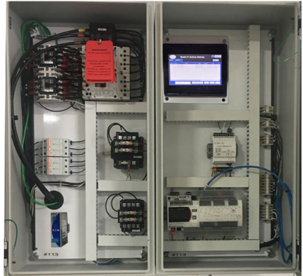
Figure 22. Module electrical and control panel
