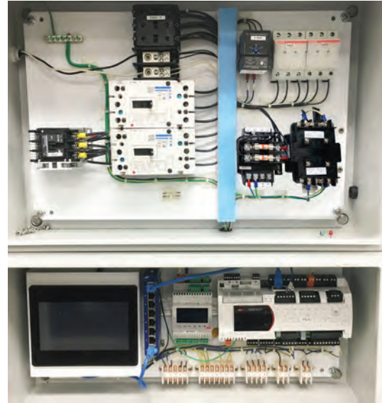
Figure 23. Module electrical and control panel
