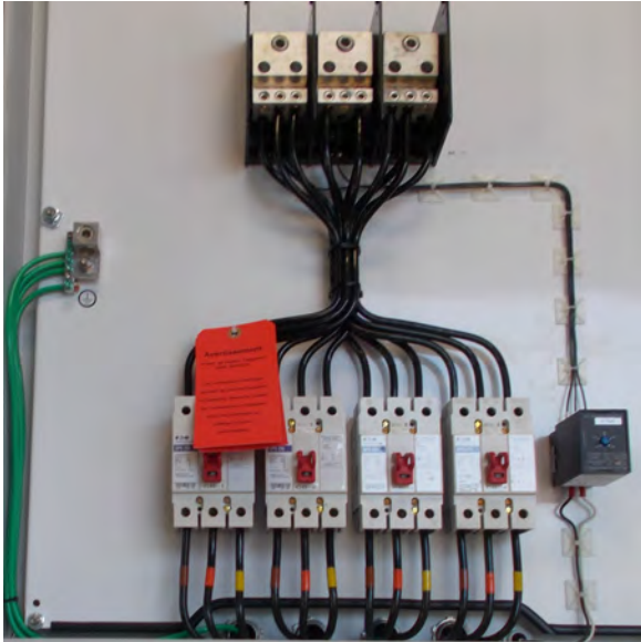
Figure 22. Power distribution panel
