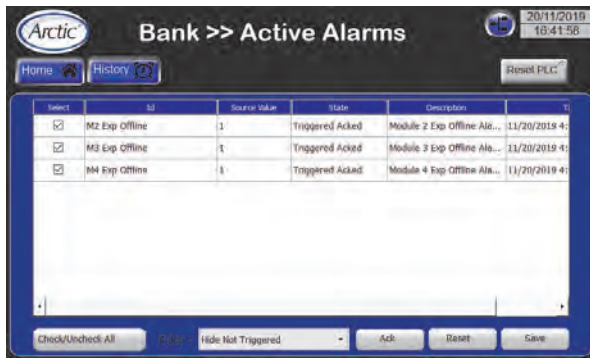
Figure 16. Active alarms for the chiller
