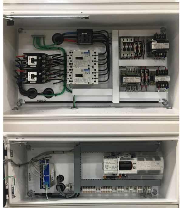
Figure 23. Module electrical panel
