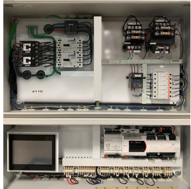
Figure 23. Module electrical and control panel
