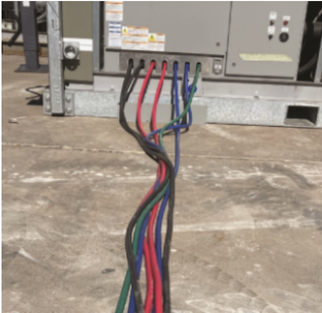
Figure 8. Incorrect installation - cable is not spaced out
