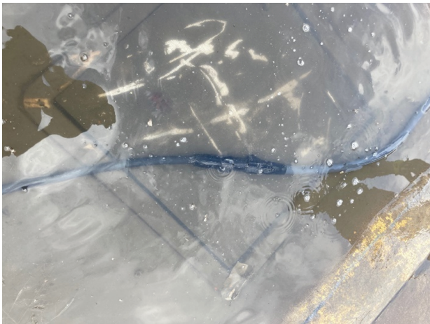
Figure 9. Incorrect installation - submerged cable
